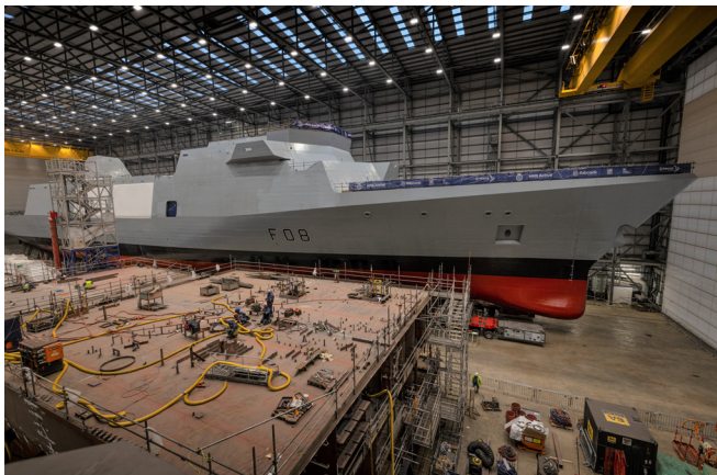
Two Type 31 ships under construction in the Rosyth Shipyard's Venturer Hall (Photo Credit: Babcock)
